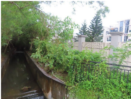
Proposed Drainage Works Area of Ha Che (CH.A 300.00 ~ CH.A 653.949) Date taken: 22 nd November 2023
